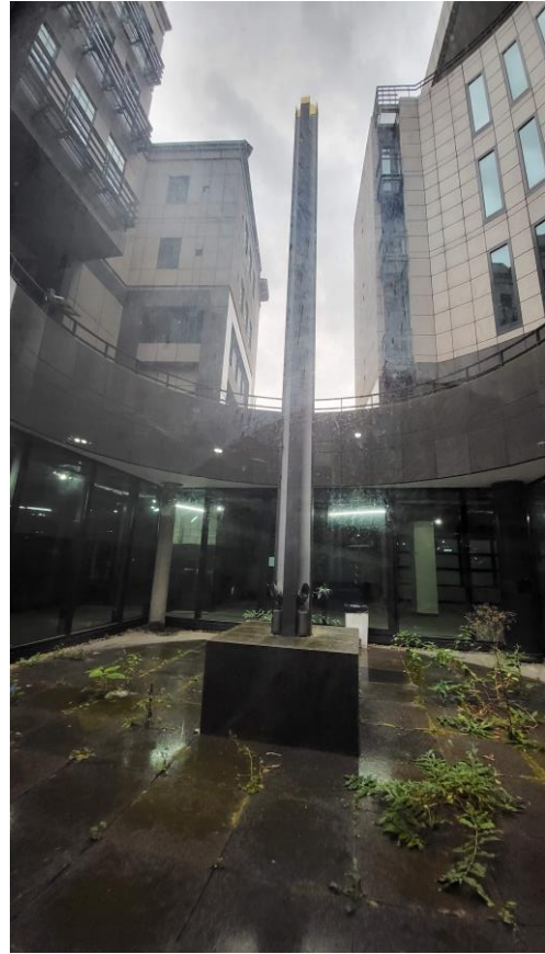
Image 7: The base of the existing lightwell in the centre of the courtyard
